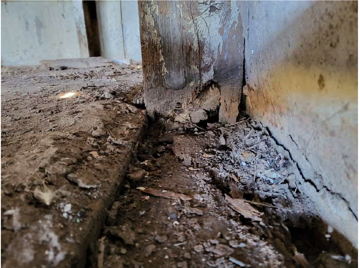
BUILDING 248 – DETERIORATION AT LOWER PORTION OF STUD WALL
