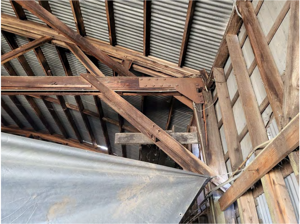
BUILDING 249 – TRUSS CONNECTION FAILURE
