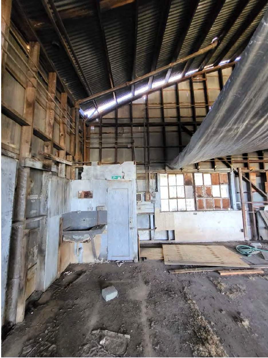
BUILDING 248 – ROOF CONNECTION DISPLACEMENT
