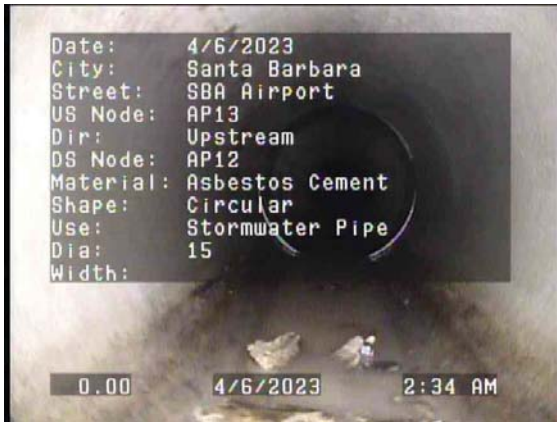
0.00ft Catch Basin / AP12
