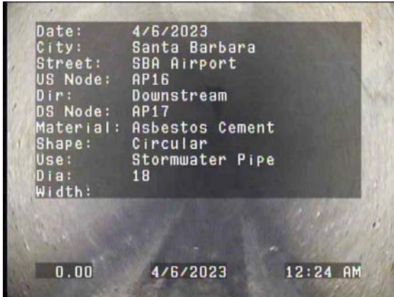
0.00ft Catch Basin / AP16
