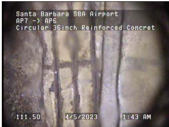
111.50ft Surface Damage Reinforcement Visible from 11 o'clock to 1 o'clock, within 8 inch
