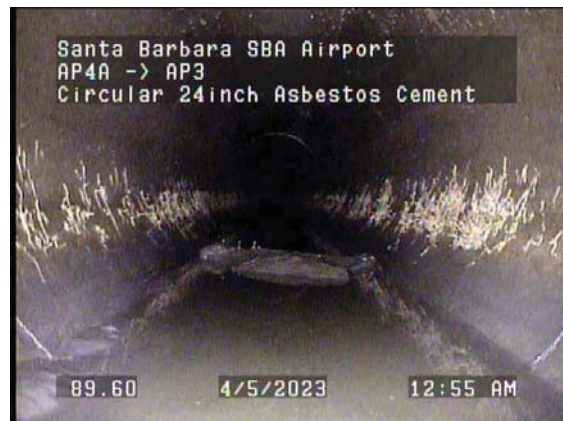
89.60ft Deposits Settled Other, 10% of cross sectional area from 5 o'clock to 7 o'clock / Debris
