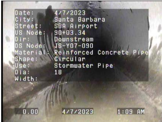
0.00ft Catch Basin / 90+03.34
