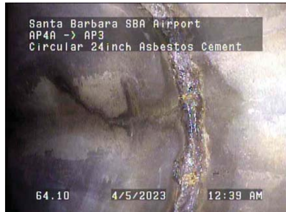
64.10ft Crack Multiple from 11 o'clock to 1 o'clock, within 8 inch
