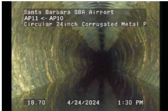
18.70ft Surface Damage Corrosion from 2 o'clock to 5 o'clock, Start
