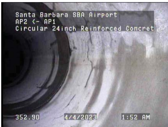
352.90ft Crack Multiple from 11 o'clock to 1 o'clock, within 8 inch
