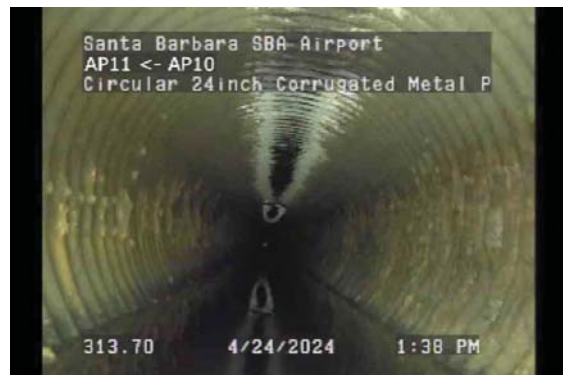
313.70ft Miscellaneous Material Change, Corrugated metal pipe / CMP
