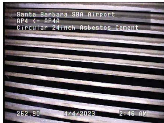
262.90ft Catch Basin / AP4
