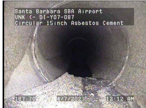
187.70ft Deposits Settled Other, 10% of cross sectional area from 5 o'clock to 7 o'clock / Debris
