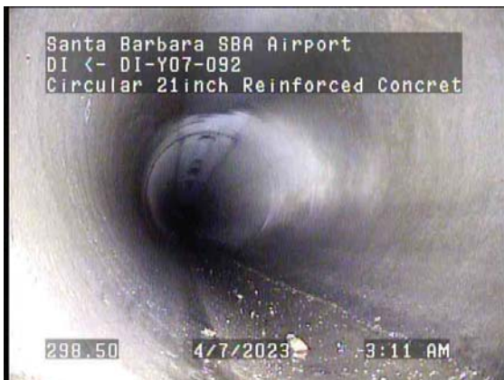
298.50ft Tap Break-in/Hammer at 9 o'clock, dia/height: 18inch
