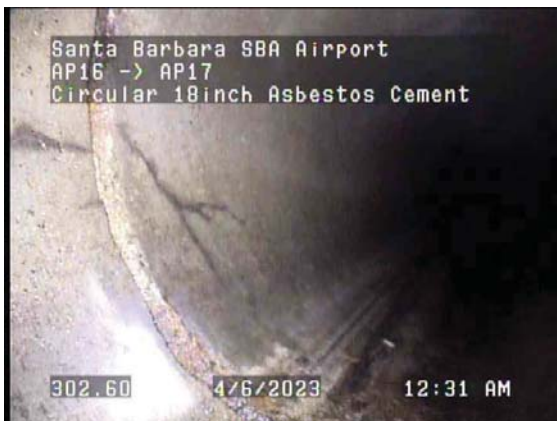
302.60ft Crack Multiple from 8 o'clock to 9 o'clock, within 8 inch
