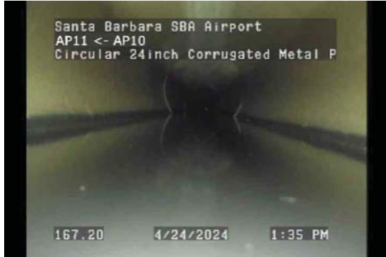
167.20ft Surface Damage Corrosion from 2 o'clock to 5 o'clock, Finish
