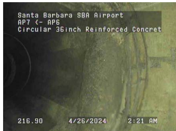
216.90ft Obstruction Intruding Through Wall, 10% of cross sectional area from 11 o'clock to 1 o'clock, within 8 inch
