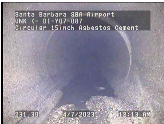
231.30ft Deposits Settled Other, 5% of cross sectional area from 5 o'clock to 7 o'clock / Debris
