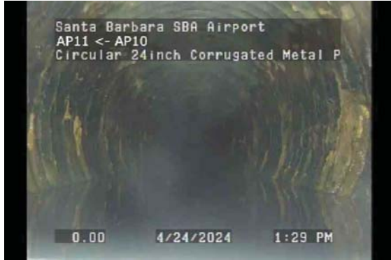
0.00ft Catch Basin / AP10
