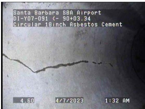
4.60ft Crack Longitudinal at 10 o'clock
