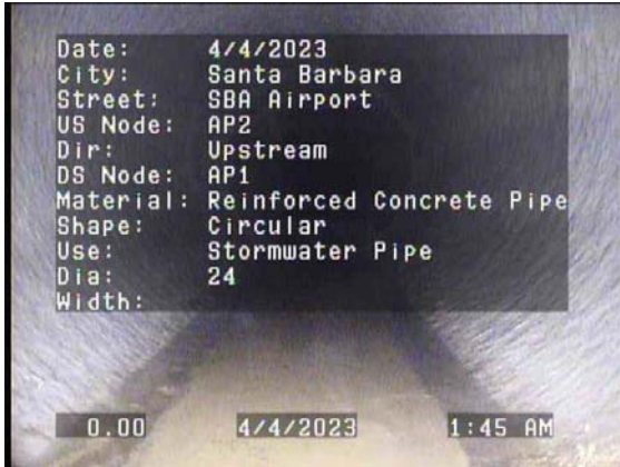
0.00ft Catch Basin / AP1
