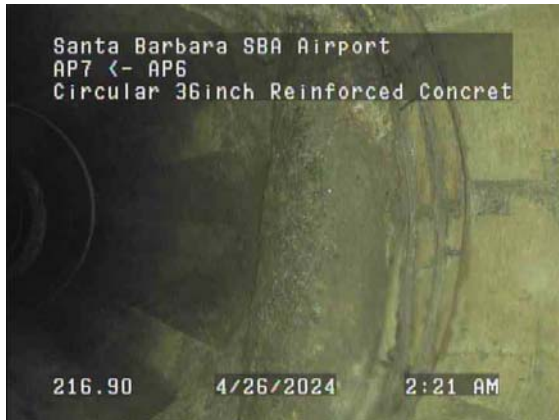
216.90ft Surface Damage Reinforcement Visible from 11 o'clock to 1 o'clock, within 8 inch
