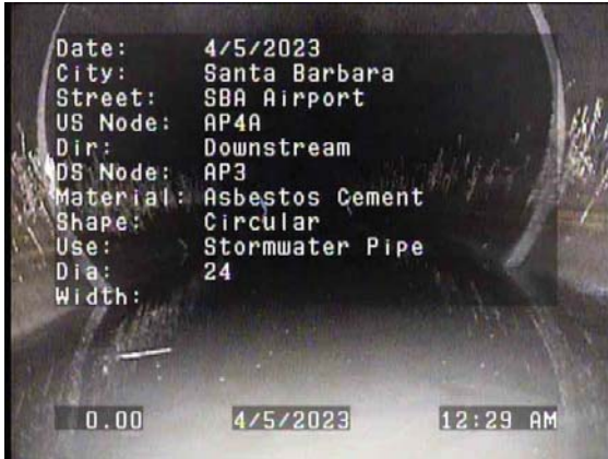
0.00ft Catch Basin / AP4A
