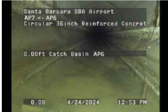
0.00ft Catch Basin / AP6
