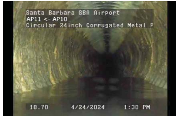
18.70ft Surface Damage Corrosion from 7 o'clock to 10 o'clock, Start
