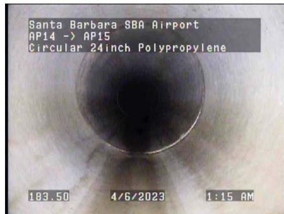
183.50ft Miscellaneous Material Change, Asbestos cement / ACP
