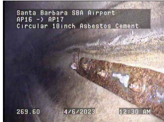
269.60ft Deposits Settled Other, 5% of cross sectional area from 4 o'clock to 5 o'clock / metal
