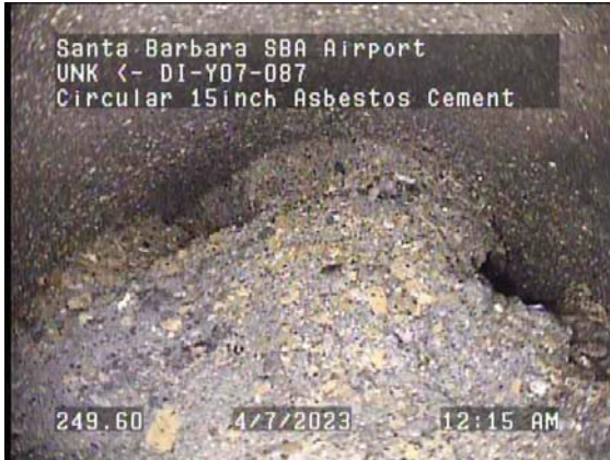
249.60ft Deposits Settled Compacted, 100% of cross sectional area from 12 o'clock to 12 o'clock / Concrete
