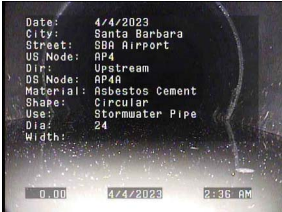
0.00ft Catch Basin / AP4A
