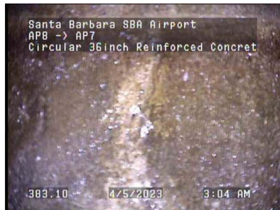
383.10ft Infiltration Runner at 4 o'clock, within 8 inch
