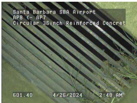
601.40ft Catch Basin / AP8
