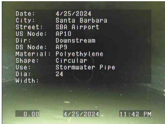
0.00ft Catch Basin / AP10
