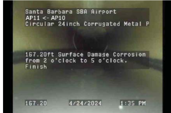
167.20ft Surface Damage Corrosion from 7 o'clock to 10 o'clock, Finish
