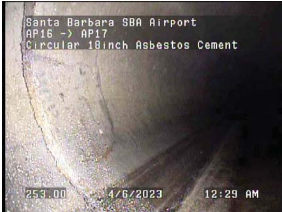
253.00ft Crack Multiple from 7 o'clock to 9 o'clock, within 8 inch
