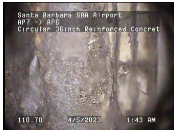
110.70ft Intruding Sealing Material Grout, 10% of cross sectional area from 11 o'clock to 1 o'clock
