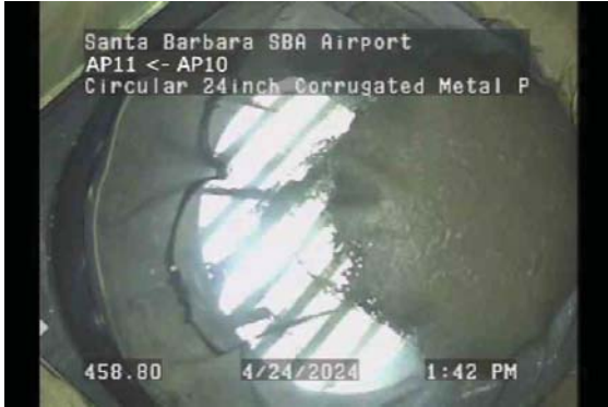
458.80ft Catch Basin / AP11
