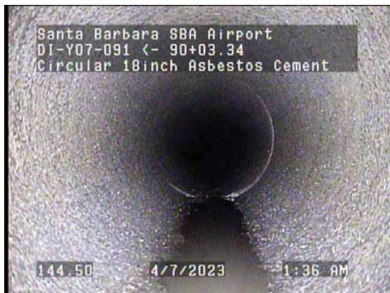
144.50ft Deposits Settled Other, 5% of cross sectional area from 5 o'clock to 7 o'clock, Finish / Debris
