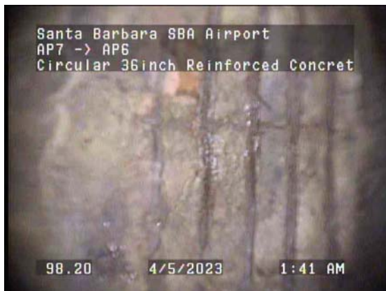
98.20ft Surface Damage Reinforcement Visible from 11 o'clock to 1 o'clock
