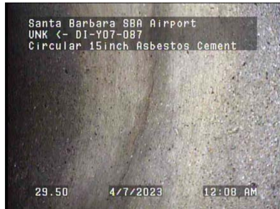
29.50ft Crack Circumferential from 7 o'clock to 5 o'clock
