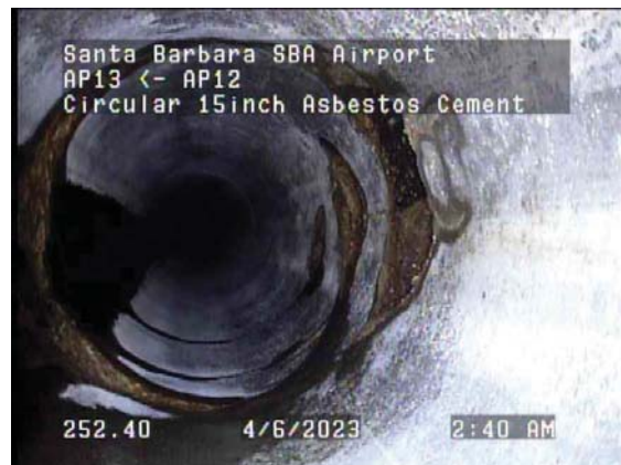
252.40ft Hole from 11 o'clock to 1 o'clock, within 8 inch
