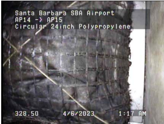
328.50ft Catch Basin / AP15
