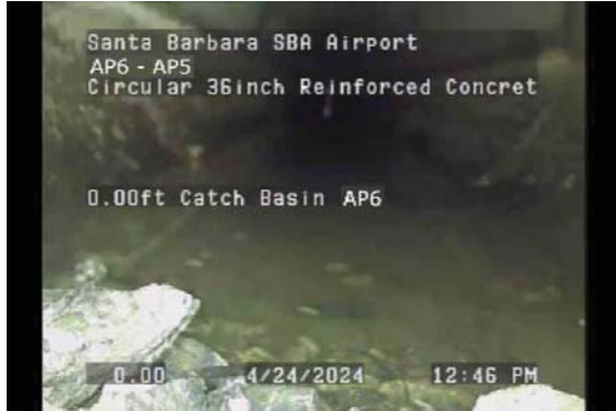
0.00ft Catch Basin / AP6
