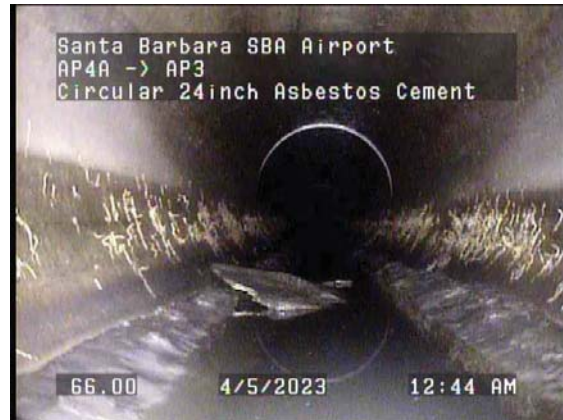
66.00ft Deposits Settled Other, 5% of cross sectional area from 6 o'clock to 7 o'clock / Debris
