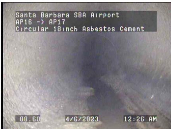
88.60ft Deposits Settled Other, 5% of cross sectional area from 5 o'clock to 7 o'clock, Start / Debris
