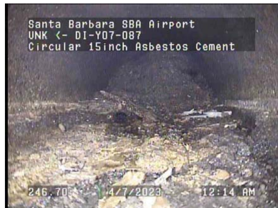
246.70ft Deposits Settled Compacted, 50% of cross sectional area from 3 o'clock to 9 o'clock / Concrete
