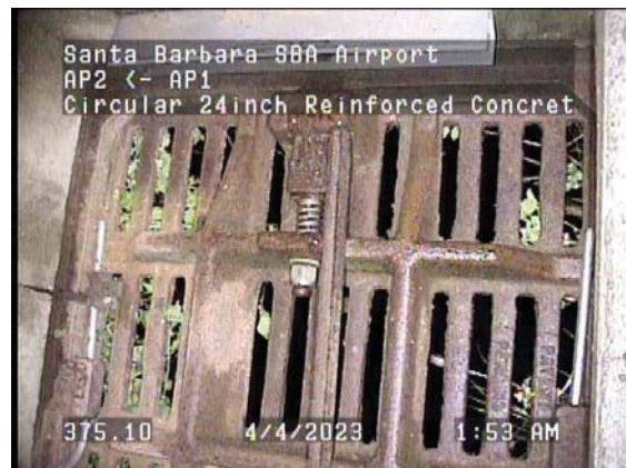
375.10ft Catch Basin / AP2
