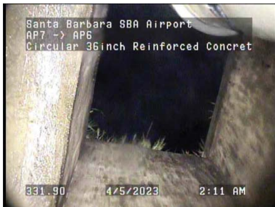
331.90ft Catch Basin / AP6
