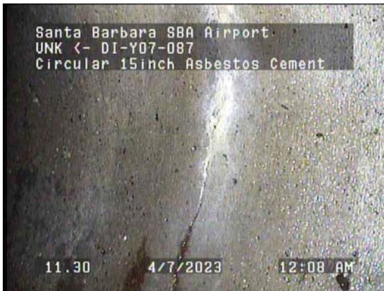
11.30ft Crack Circumferential from 7 o'clock to 5 o'clock
