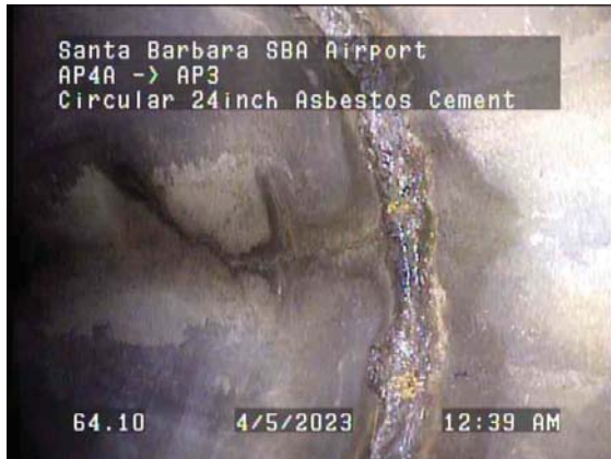
64.10ft Infiltration Dripper at 12 o'clock, within 8 inch
