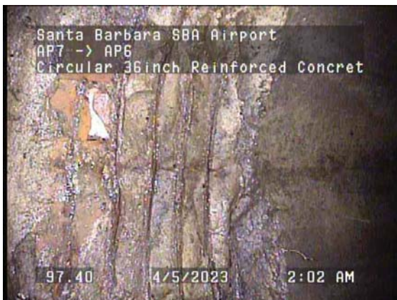
97.40ft Surface Damage Reinforcement Visible from 11 o'clock to 1 o'clock, within 8 inch
