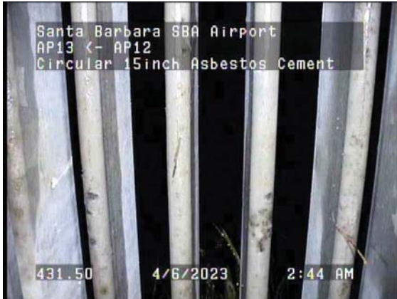
431.50ft Catch Basin / AP13
