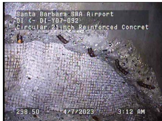
298.50ft Surface Damage Reinforcement Visible from 9 o'clock to 10 o'clock
