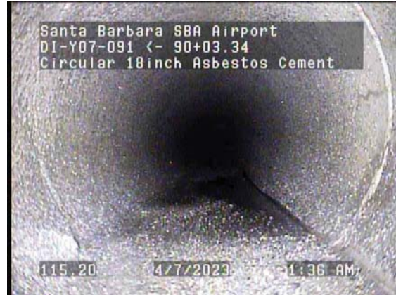
115.20ft Deposits Settled Other, 5% of cross sectional area from 5 o'clock to 7 o'clock, Start / Debris
