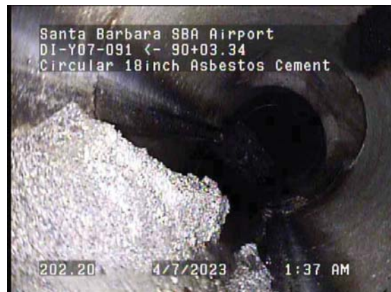
202.20ft Deposits Settled Other, 10% of cross sectional area from 5 o'clock to 7 o'clock / Debris
