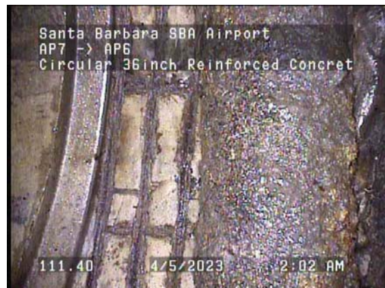
111.40ft Surface Damage Reinforcement Visible from 11 o'clock to 1 o'clock, within 8 inch
