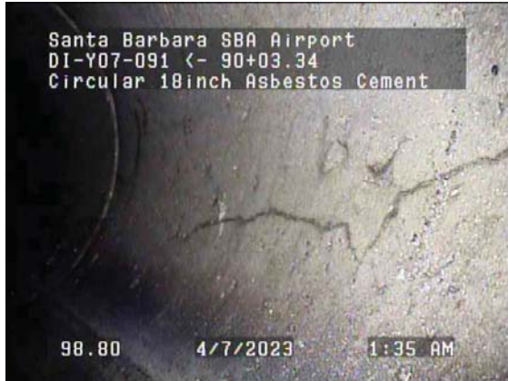
98.80ft Crack Multiple from 3 o'clock to 4 o'clock
